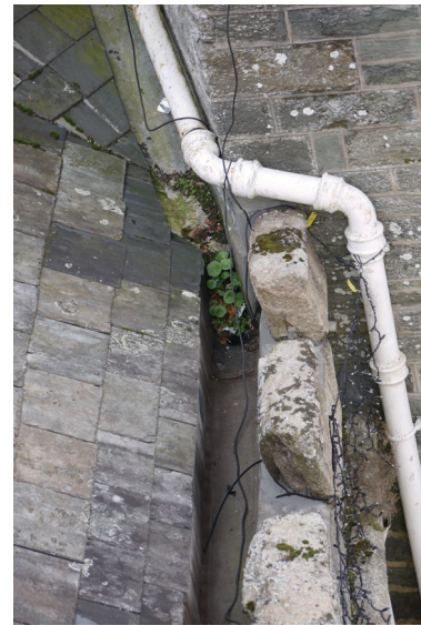
EXISTING PHOTO - POLICE STATION GUTTER Existing gutter with bituminous render and asphalt gutters 1:5 @ A1
