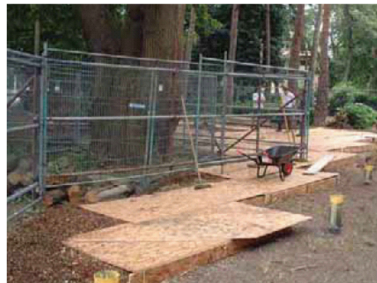
Figure A1.02 - Ground spreader boards atop of a compressible layer of woodchip.
