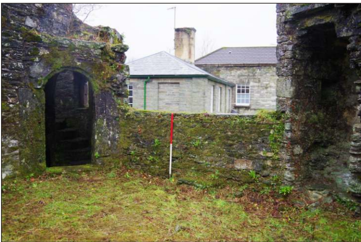
Plate 22: West elevation of first-floor room above the gate-hall of Betsy Grimal's Tower, looking east. (1m scale)
