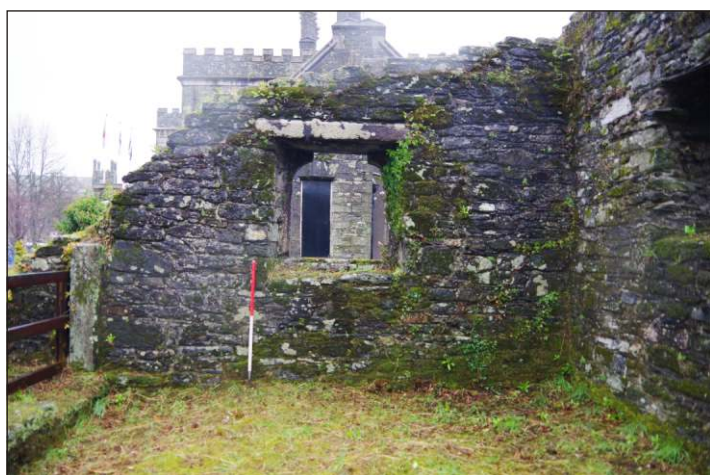
Plate 20: East elevation of first-floor room above the gate-hall of Betsy Grimbal's Tower, looking east-northeast. (1m scale)
