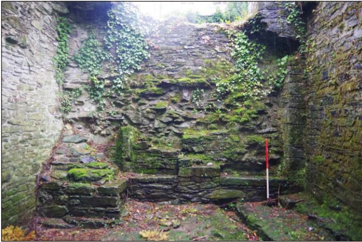
Plate 11: East elevation of north wing of Betsy Grimal's Tower, looking south-southeast. (1m scale)
