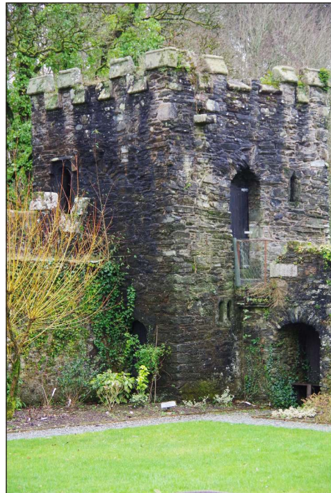
Plate 30: North and east elevations of the Still House, looking south. (1m scale)
