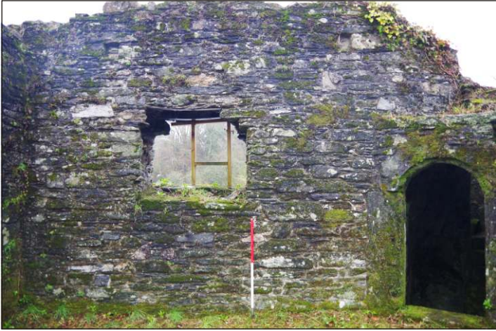
Plate 21: South elevation of first-floor room above the gate-hall of Betsy Grimal's Tower, looking south-southeast. (1m scale)
