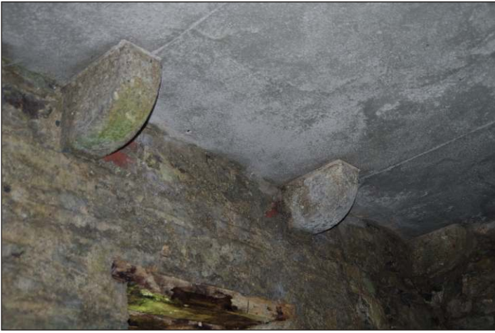
Plate 39: Detail of first-floor corbels on west elevation of the Still House, looking east. (1m scale)
