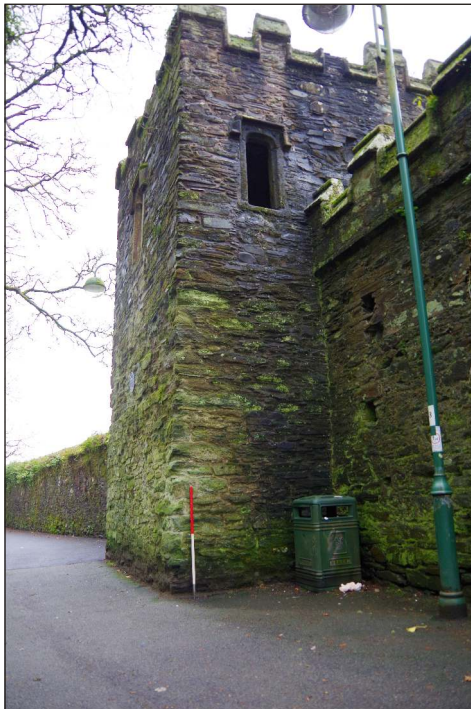
Plate 29: East and south elevations of the Still House, looking north-northwest. (1m scale)
