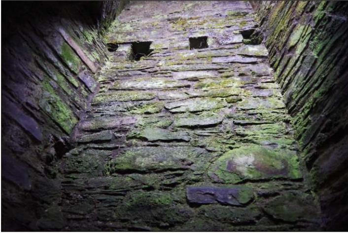
Plate 24: Joist sockets in north turret for first-floor of Betsy Grimal's Tower, looking west-southwest
