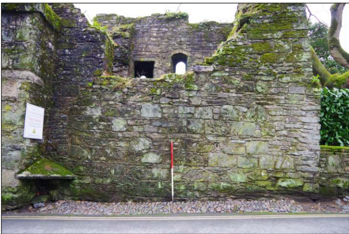
Plate 5: North end of the east elevation of Betsy Grimal's Tower, looking west-southwest. (1m scale)
