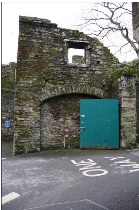
Plate 6: South end of the east elevation of Betsy Grimal's Tower, looking west-southwest. (1m scale)
